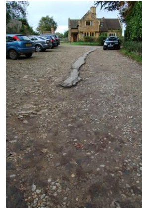
Figure 23: Road surface at Churchfields
